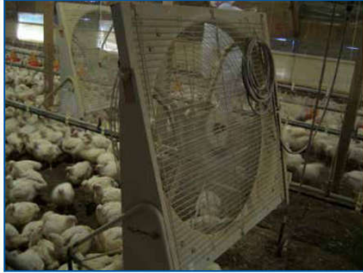
شكل (154) Circulation fans in a naturally ventilated house
