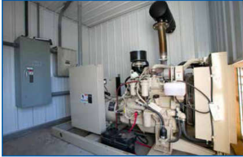
شكل (151) Example of a back-up generator
