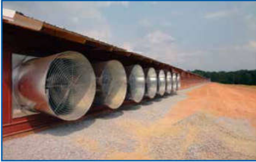
شكل (٤٣) Example of a typical tunnel ventilated house
